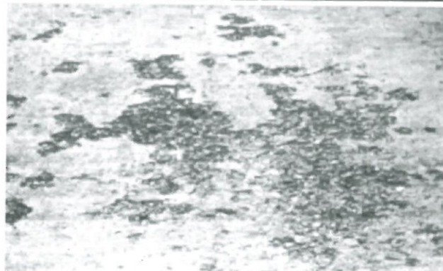
Scaling concrete surface
