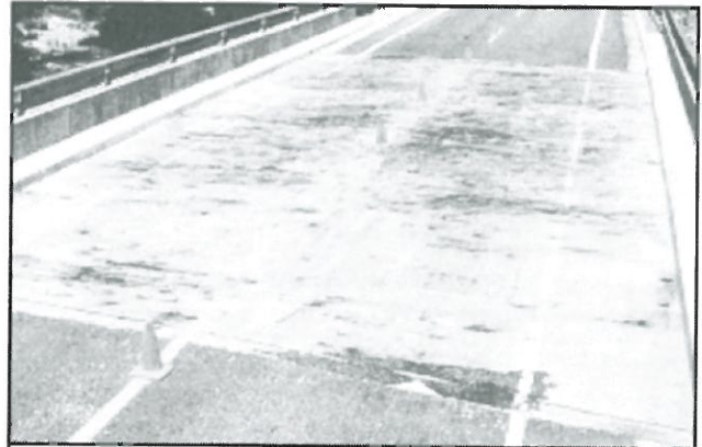
Steel corrosion on a bridge deck
