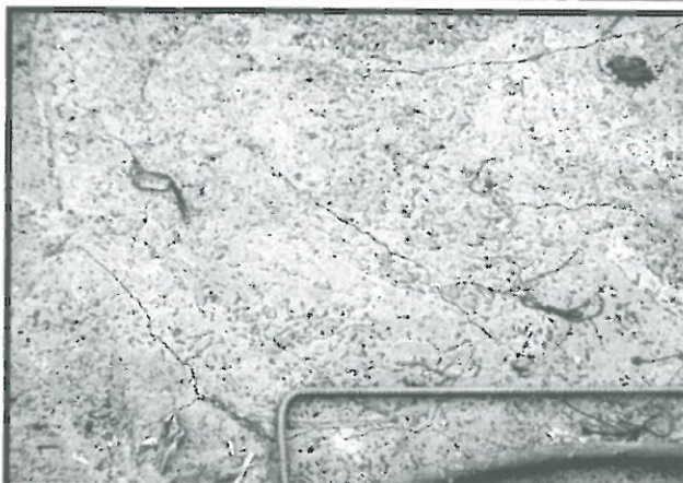
Thermal cracks in a thick slab
